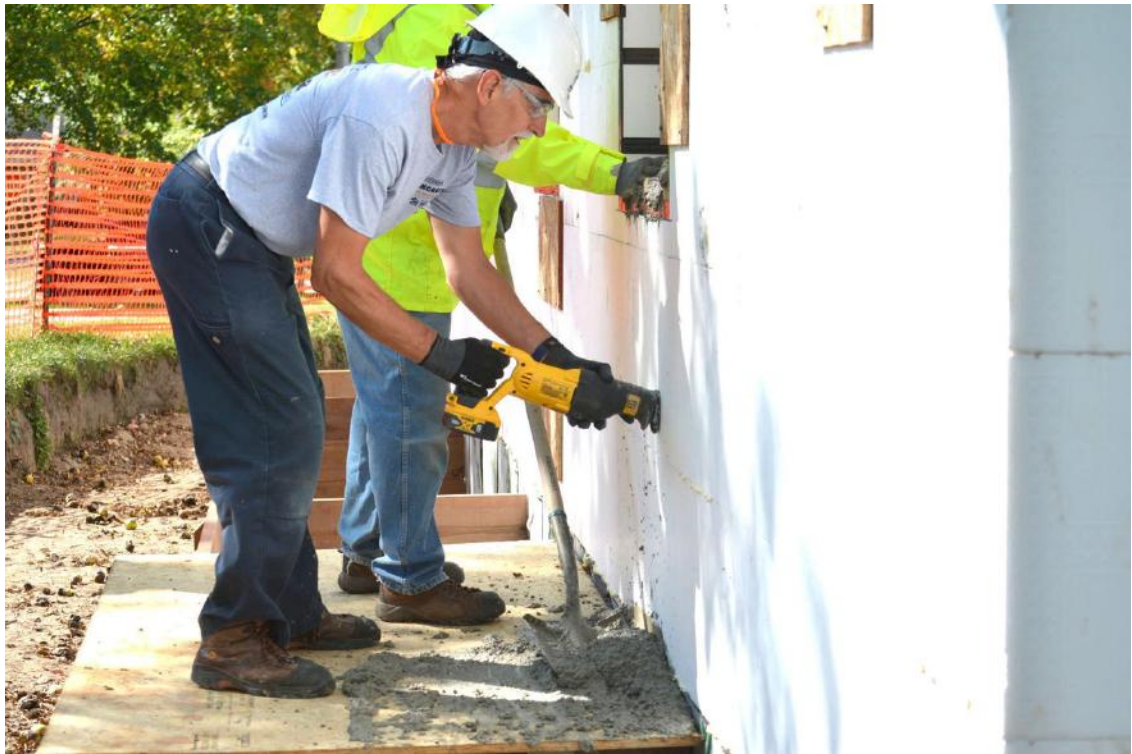
Habitat for Humanity volunteer Dave Wolf helps construct what will become the Strand family home in Northfield on Tuesday. Wolf is using a reciprocating blade inserted, to help settle concrete as it is poured into forms. (Zach Kayser/southernminn.com)
